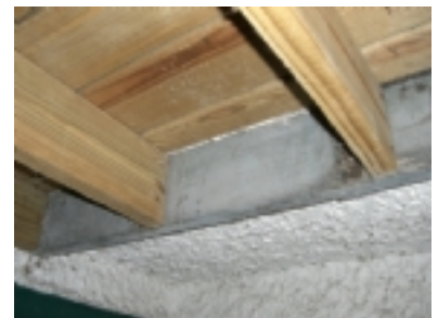
Picture Date:10/26/2006 Comments: No joist hangers installed.
