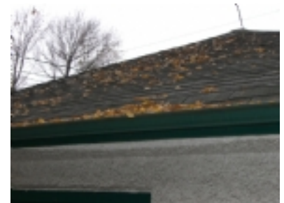
Picture Date:10/26/2006 Comments: Gutters clogged with leaves.
