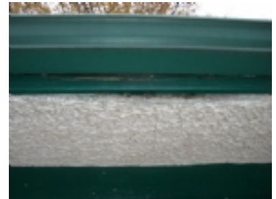
Picture Date:10/26/2006 Comments: Soffit on garage is loose.
