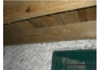
Picture Date:10/26/2006 Comments: Ledger board has only been nailed. Lag bolts should be used to fasten ledger to house.
