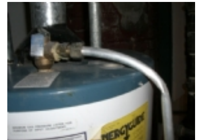
Picture Date:10/26/2006 Comments: Pipe is too small and has a kink in it.
