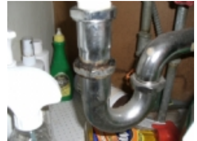
Picture Date:10/26/2006 Comments: Corroded trap
