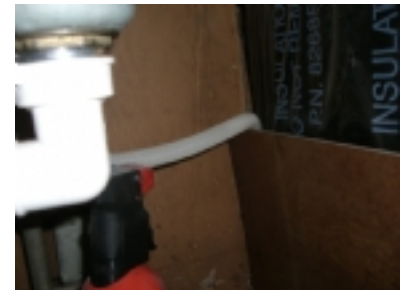
Picture Date:10/26/2006 Comments: Smaller white plastic pipe to the right should have a loop in it and be above the drain on the sink to prevent water from draining back into the dish washer.
