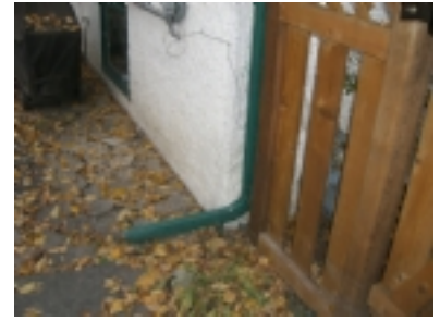
Picture Date:10/26/2006 Comments: downspout is draining too close to the house.
