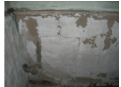
Picture Date:10/26/2006 Comments: Cracks in foundation wall in basement.
