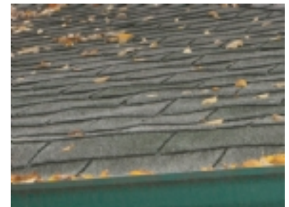
Picture Date:10/26/2006 Comments: Curled roofing
